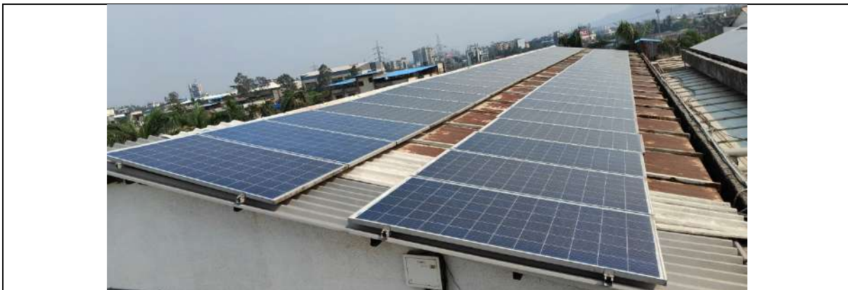
Fig. 1 Photograph of solar panels
